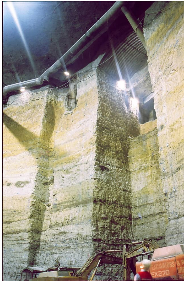
Figure 5: Near the base of the excavation, showing the sidewall slot that contains the lifts and stairs
