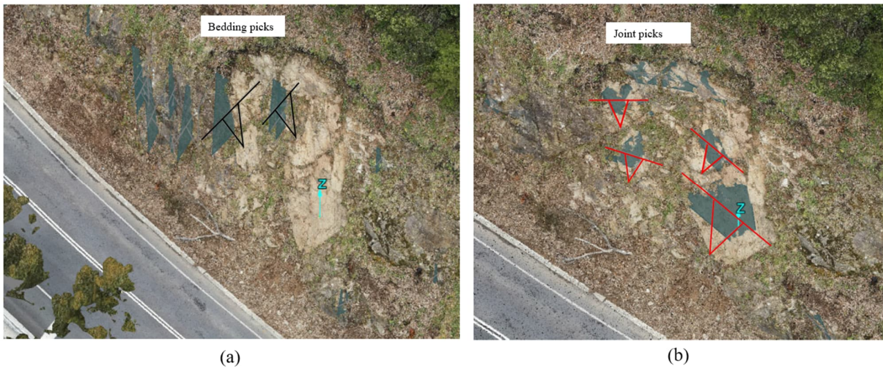
Figure 15: Photogrammetry picks at the Ch. 85 wedge failure (a) bedding planes (b) joint planes
