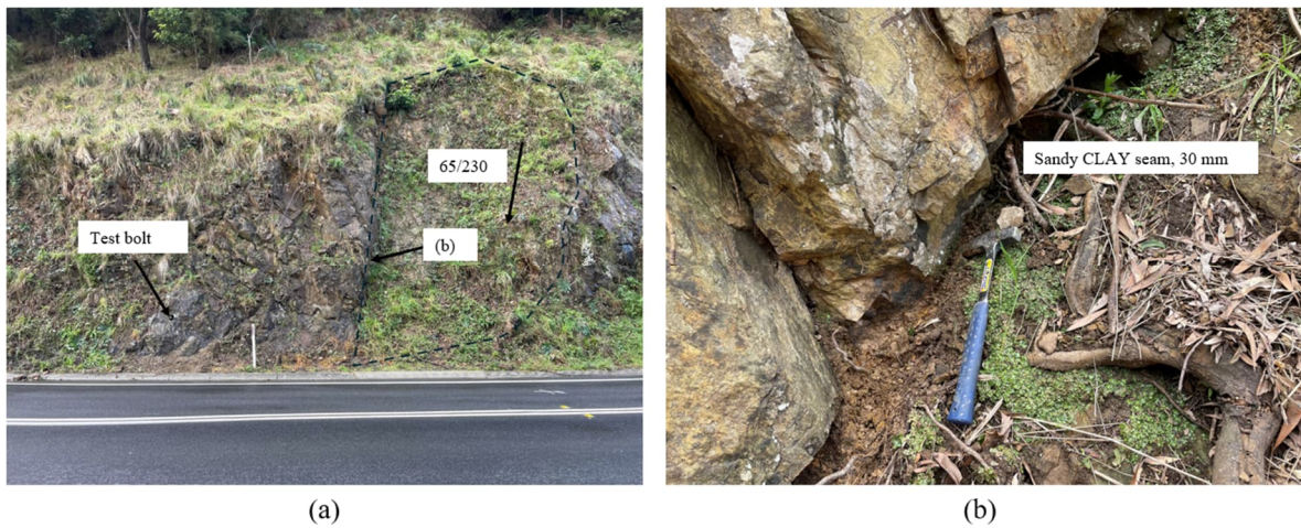
Figure 11: Planar slide at Ch. 115 of Figure 12. (a) Test bolting location and extent of failure (b) Sandy CLAY seam identified as the infill on the sliding plane
