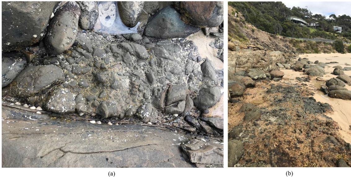
Figure 8 (a): Fault with re-cemented boulders/cobble infill which strikes sub-parallel to the gully. Location is highlighted in blue in Figure 3. (b) Looking along strike of the fault towards the GOR and Morley Avenue properties
