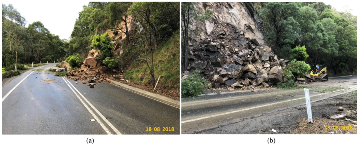
Figure 9: Excerpt from DTP failure records from 18 August 2018 (a) Looking north (b) Looking east
