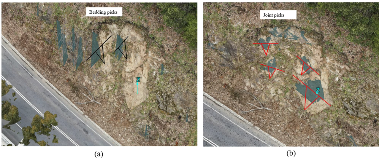
Figure 15: Photogrammetry picks at the Ch. 85 wedge failure (a) bedding planes (b) joint planes
