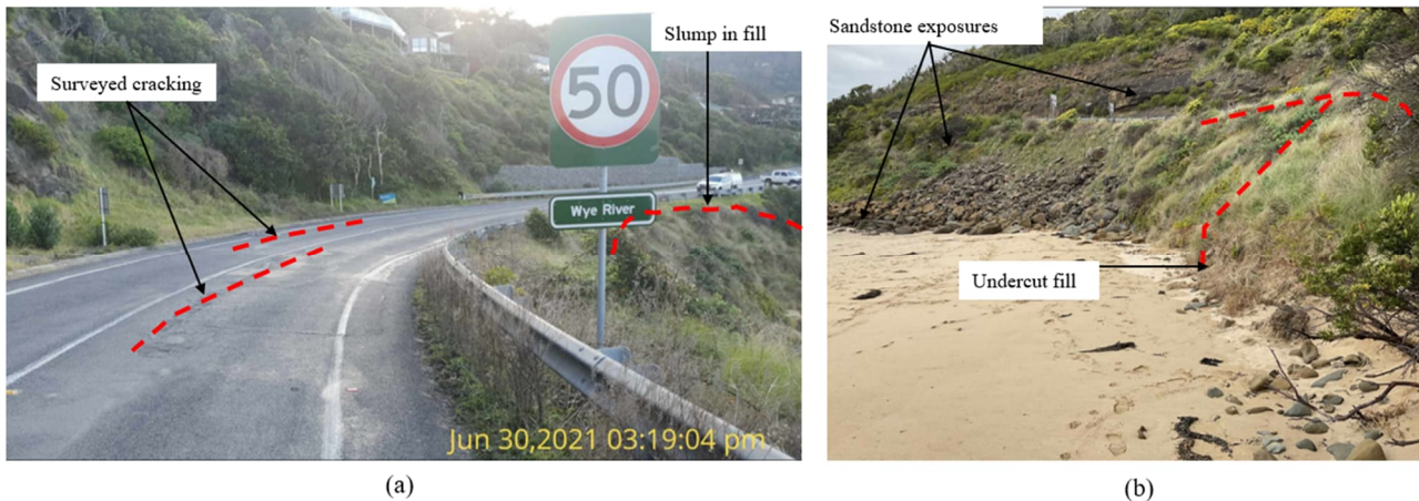
Figure 2: (a) Pavement cracking in proximity to fill failure looking towards Morley Avenue (b) Looking south towards the Wye River headland with undercut fill slope highlighted
