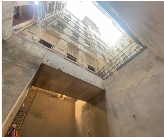
Figure 17: Photograph of the completed transfer structure, taken from the bottom of the shaft
