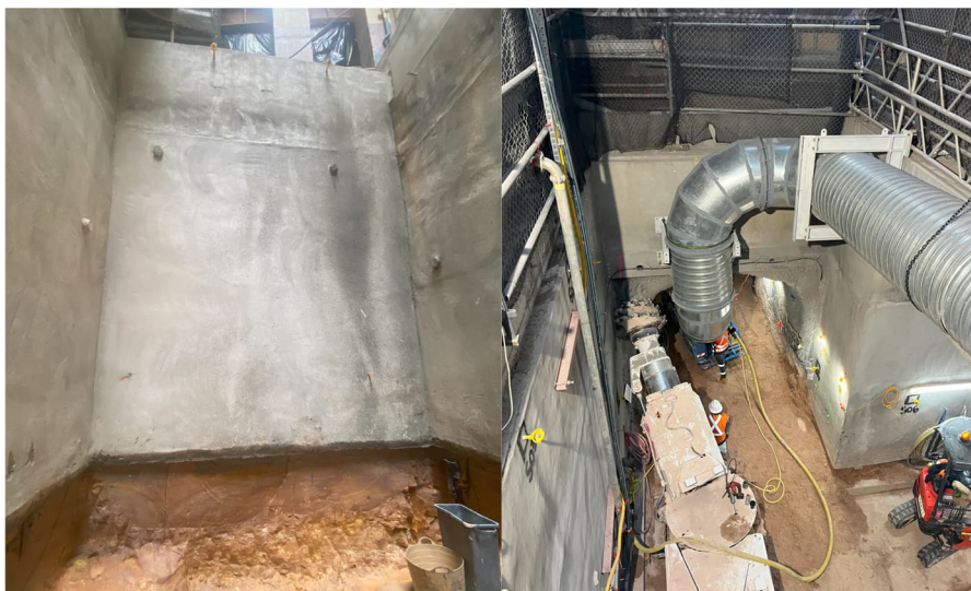
Figure 18: Photograph of the completed tunnel portal before tunnel breakthrough (left) and after tunnel breakthrough (right)
