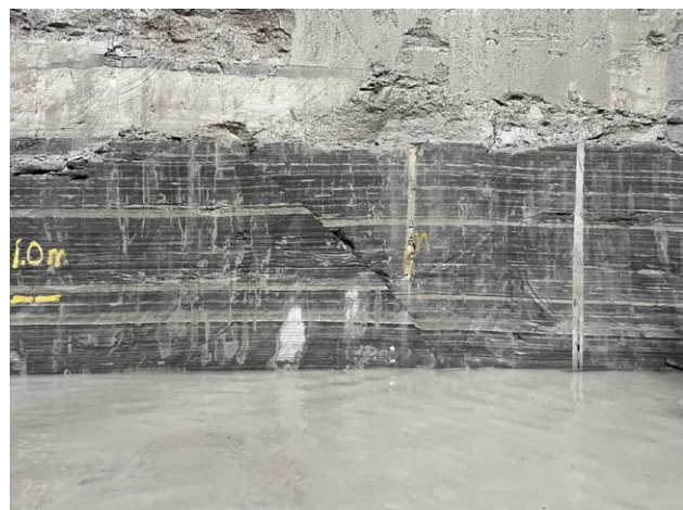
Figure 8: Localised fault within the laminite bed along the southern elevation
