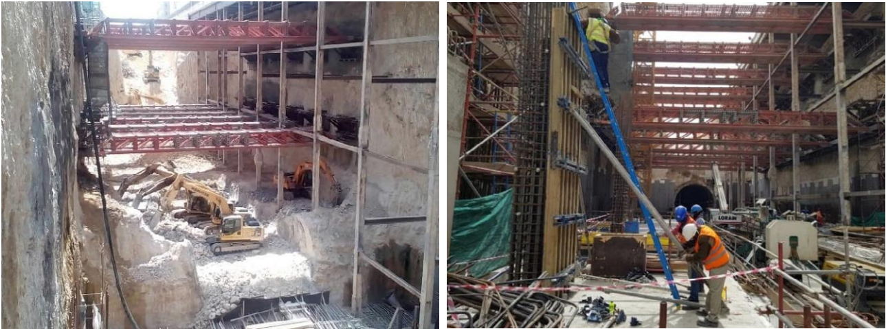
Figure 4: Left – Excavation about 2m above excavation bottom; Right – base slab already casted
