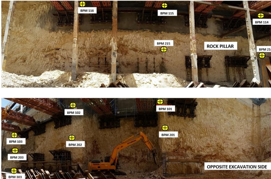
Figure 15: Monitoring prisms – rock pillar (top) and excavation opposite side (bottom) (upper props installed; brackets for support of lower props being installed)
