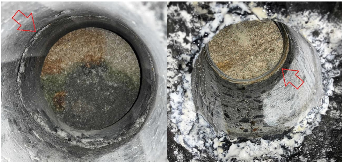
Figure 1: Examples of delamination zones evident in core holes a) inside shotcrete, and b) at the shotcrete/substrate boundary, leading to zero bond strength results.
