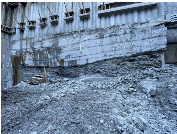
Figure 7: Upper shear zone exposed along the northern elevation
