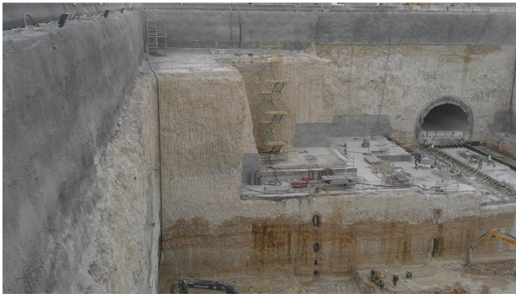
Figure 5: Another station excavation (30 m depth) in similar rock type (Breccia Limestone) and quality
