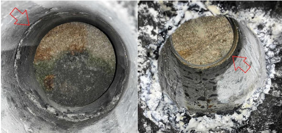
Figure 1: Examples of delamination zones evident in core holes a) inside shotcrete, and b) at the shotcrete/substrate boundary, leading to zero bond strength results.
