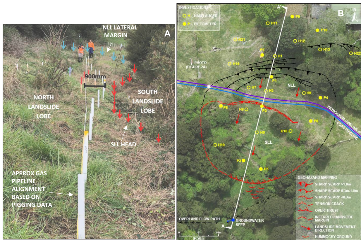
Figure 2: (A) Photo facing east across the landslide showing the inferred downslope deflection from assumed as-built alignment of the gas pipeline. (B) Simplified engineering geology sketch plan. Section A-A' shown on Figure 3.
