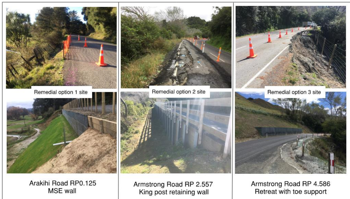
Figure 5: Examples showing the initial storm damage and final constructed design for each remedial option.
