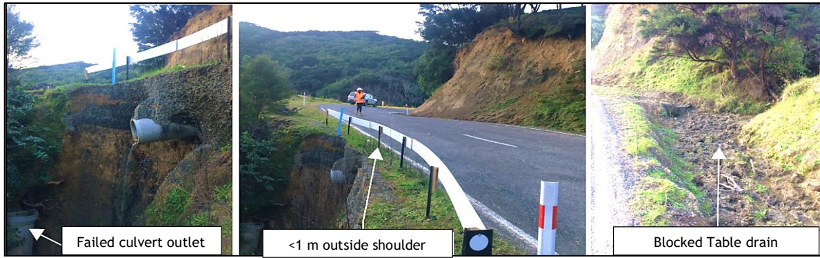
Figure 4: Anaura Road RP6.18 – Example site of scour from uncontrolled stormwater.
