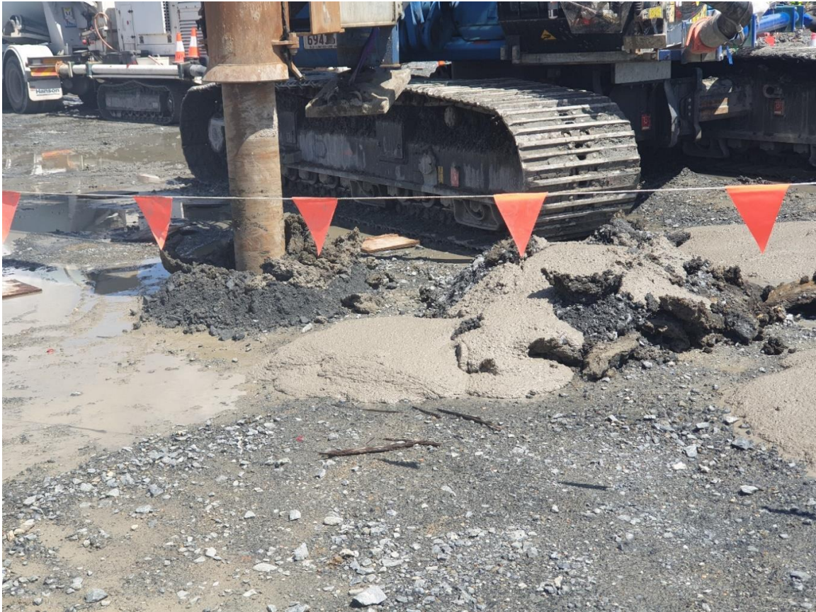
Figure 3: Heaving of wet concrete during installation of an adjacent CMC
