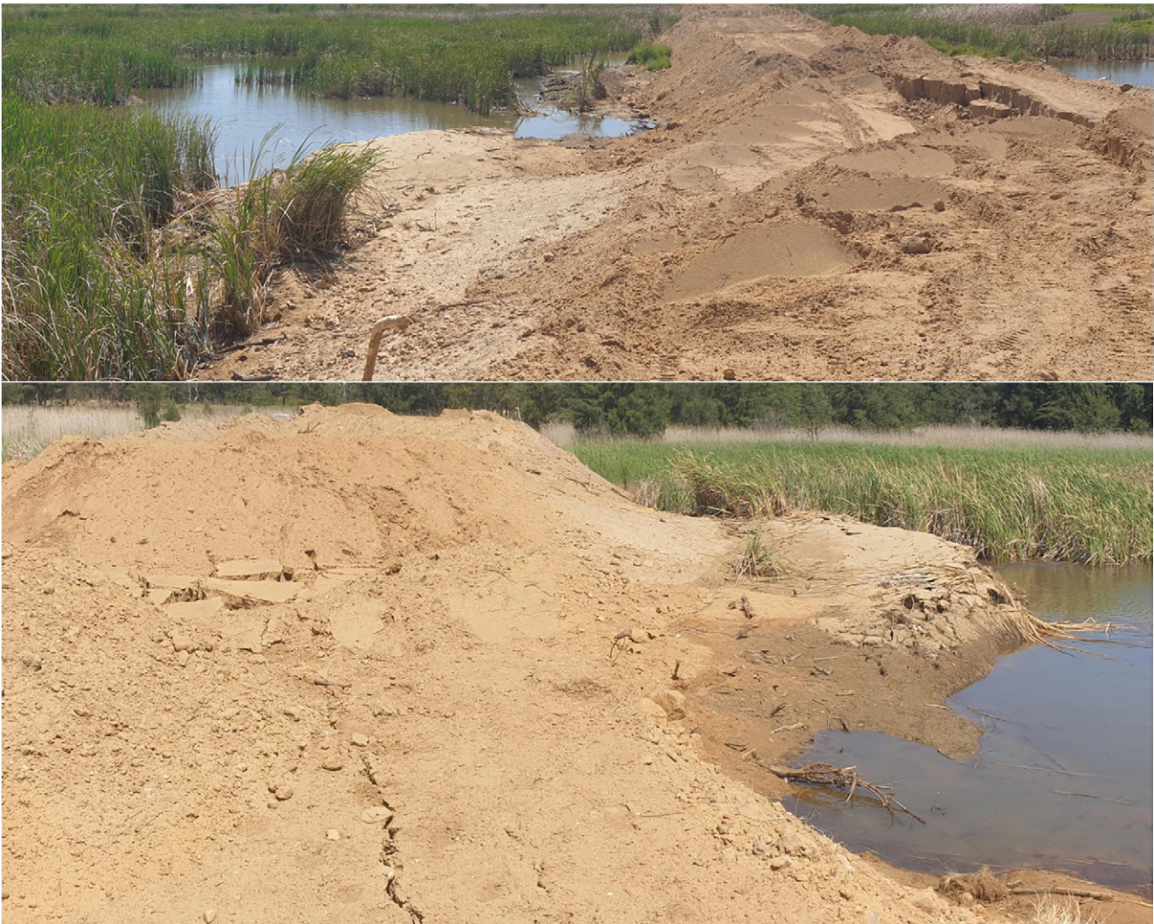
Figure 11: Formation of “mud wave” and local instability during construction
