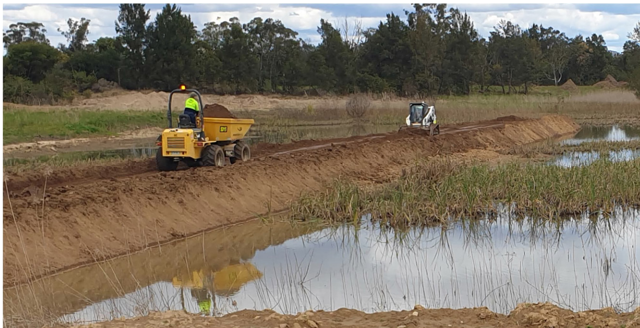
Figure 12: Revised plants with the construction of one of the bunds and some mud-waving halfway along.
