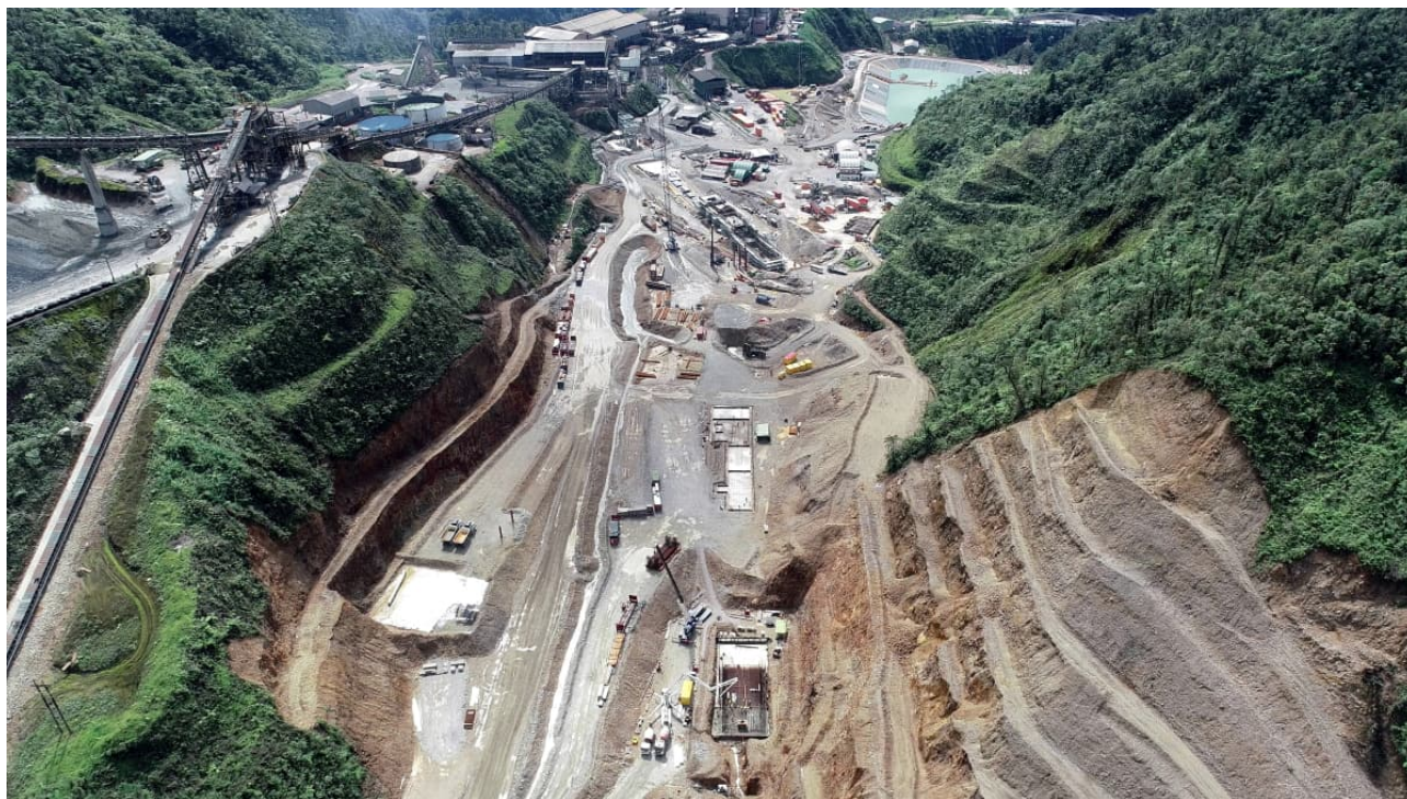
Figure 16: Overview of the TSF, with filling complete, and the new infrastructure under construction
