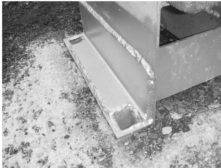
Figure 2. The steel base plates required thickening following the strengthening of the foundation (at alternative ends of the flying fox). The large weld on the base plate is the results of this thickening.
