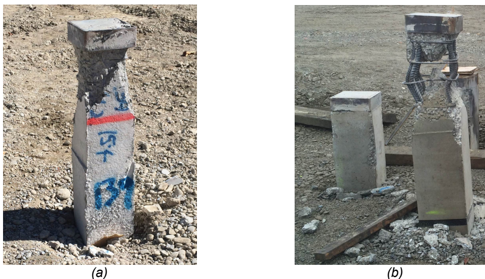
Figure 1. Pile damage to a pile that was (a) driven to the target depth range; and (b) refused above the target depth range
