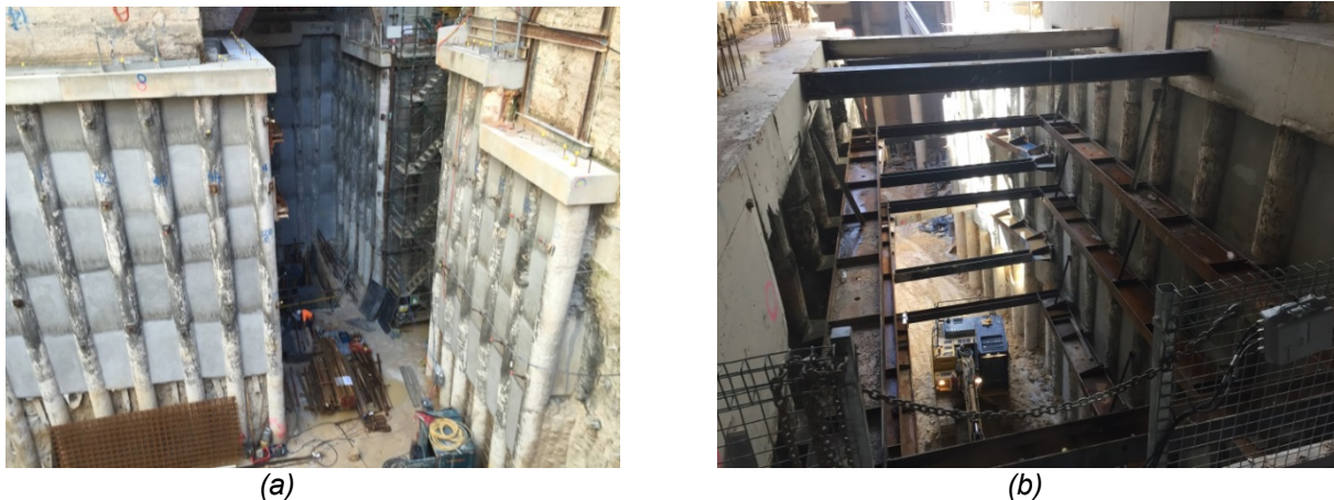
Figure 3. View of excavation faces for the York and George Street project – (a) York and George, Sydney – Carlton House; and (b) York and George, Sydney – Spiden House
