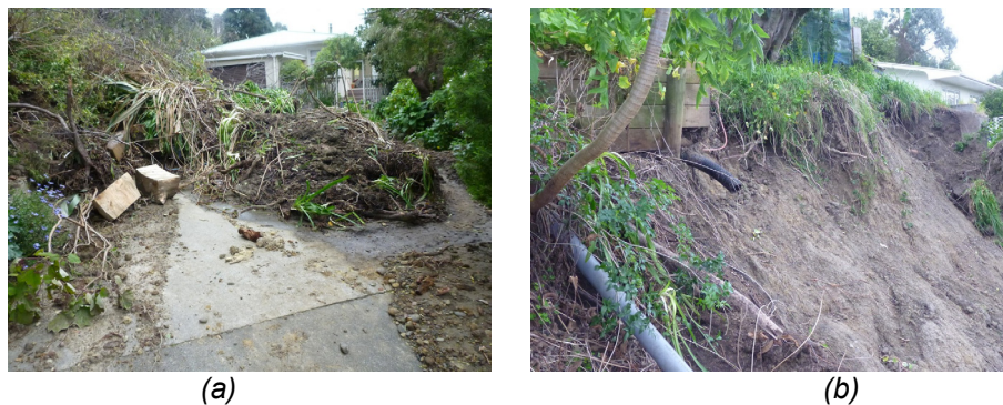
Figure 2. Photographs of the damage observed during the reconnaissance in early July 2015. (a) Debris which had inundated dwelling and accessway; and (b) landslip headscarp observed within a few metres of a dwelling.
