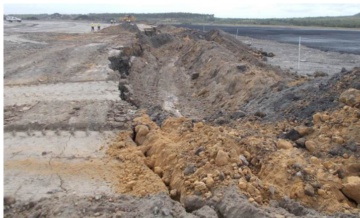
Figure 1. Large scale slip failure during capping works at a NSW coal mine
