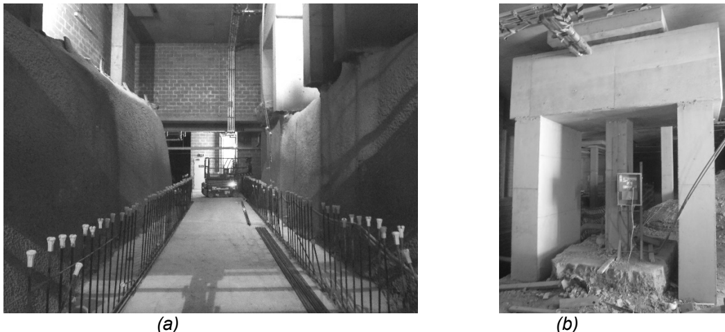
Figure 6. (a) The excavated egress tunnel looking north; and (b) a completed headstock and pair blade walls
