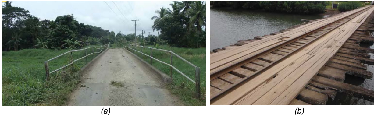
Figure 2. View of the old bridges: (a) Vunivaivai bridge and (b) Cogeloa Bridge.
