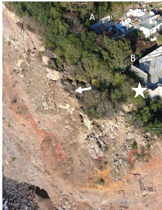
Figure 3(b). 65 – 85 m high sea cliff below A and B Whitewash Head, Scarborough. Note: missing timber-framed lookout, vegetation, and visible crack sub-parallel to cliff face (14/06/2016 Aurecon).
