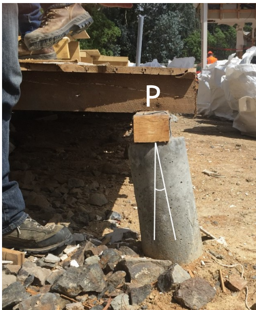
Figure 5(a). Tilted >10^\circ concrete pile (P) on Property A (18/02/2016 Aurecon).
