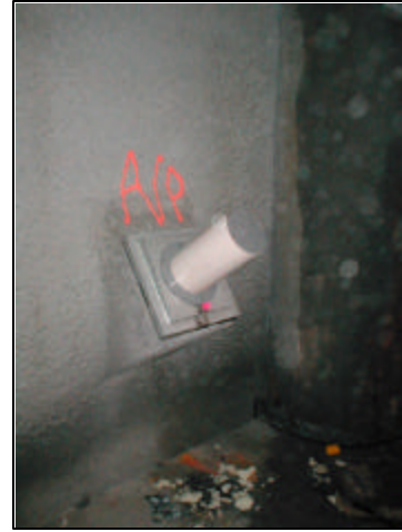
Figure 9 – Grease capped RES anchor
