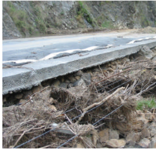
Photograph 2 Damage to pavement due to the migration of fine material.
