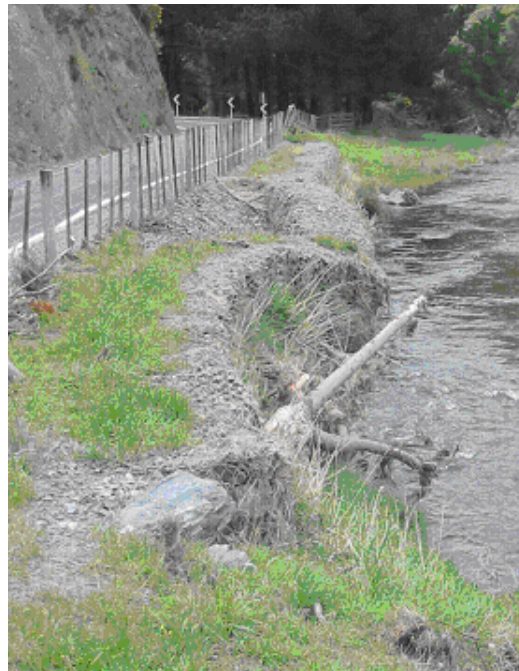
Photograph 4 Gabion wall where the middle section has been undermined and rotated.
