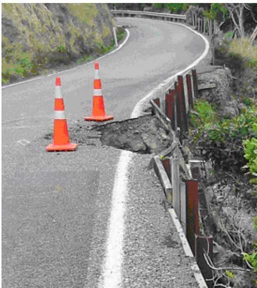
Photograph 3 Undermined railway iron wall with loss of backfill material.
