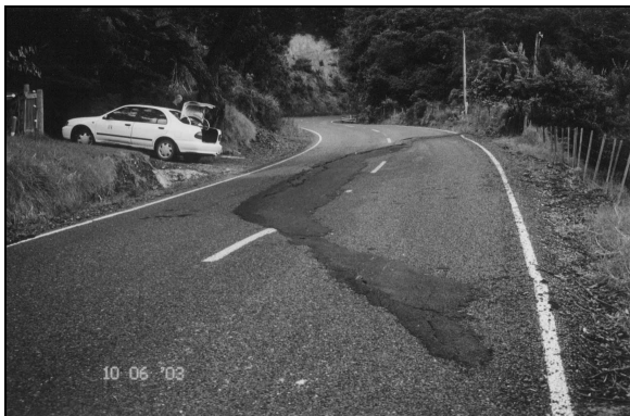
Photo 1. Head Scarp of Slip on evening of 10 June 2003
