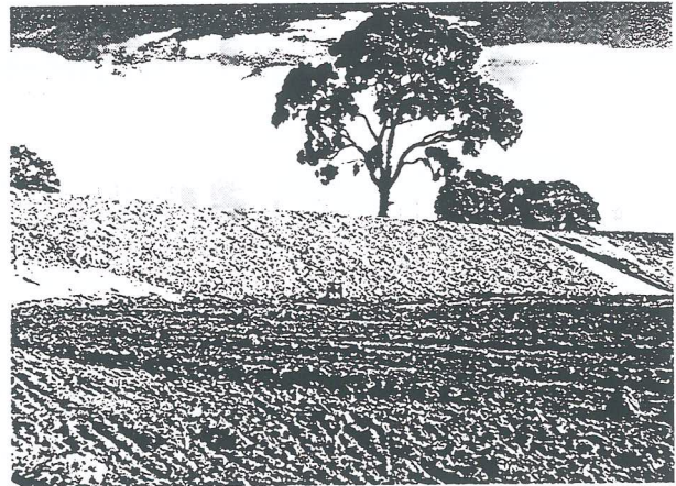
Figure 4: placement of rip rap rock over the Bidim A24 geofabric filter cloth.
