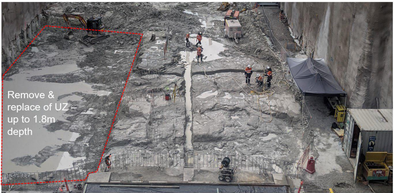
Figure 23: Excavation of Unconformity Zone materials for the Boggo Road Station invert floor treatment.
