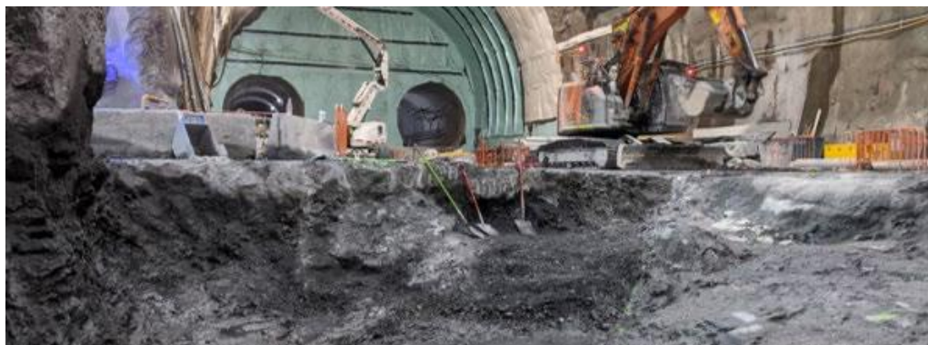
Figure 18: Excavation of fault materials for the Albert Street Station cavern invert floor treatment.
