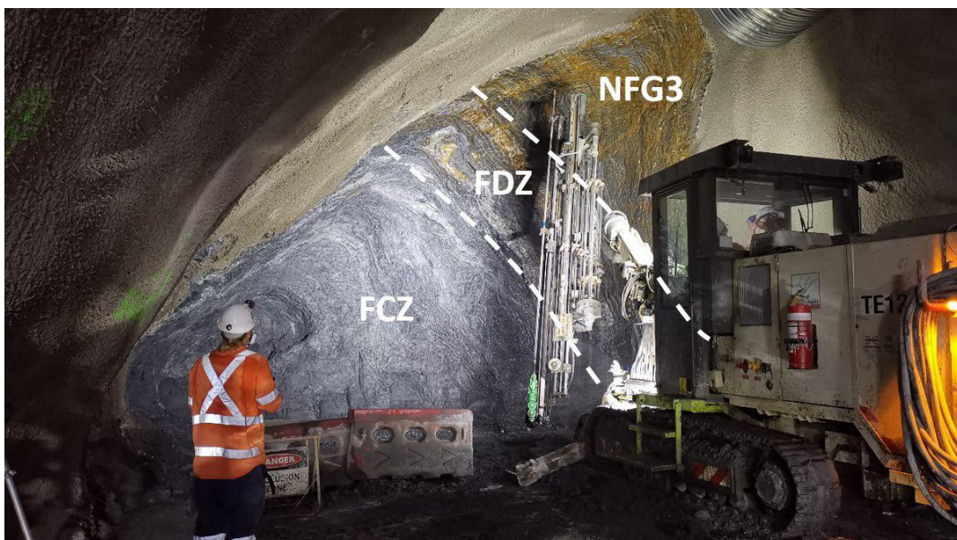
Figure 8: Fault zone encountered in the Roma Street Station cavern heading during construction.
