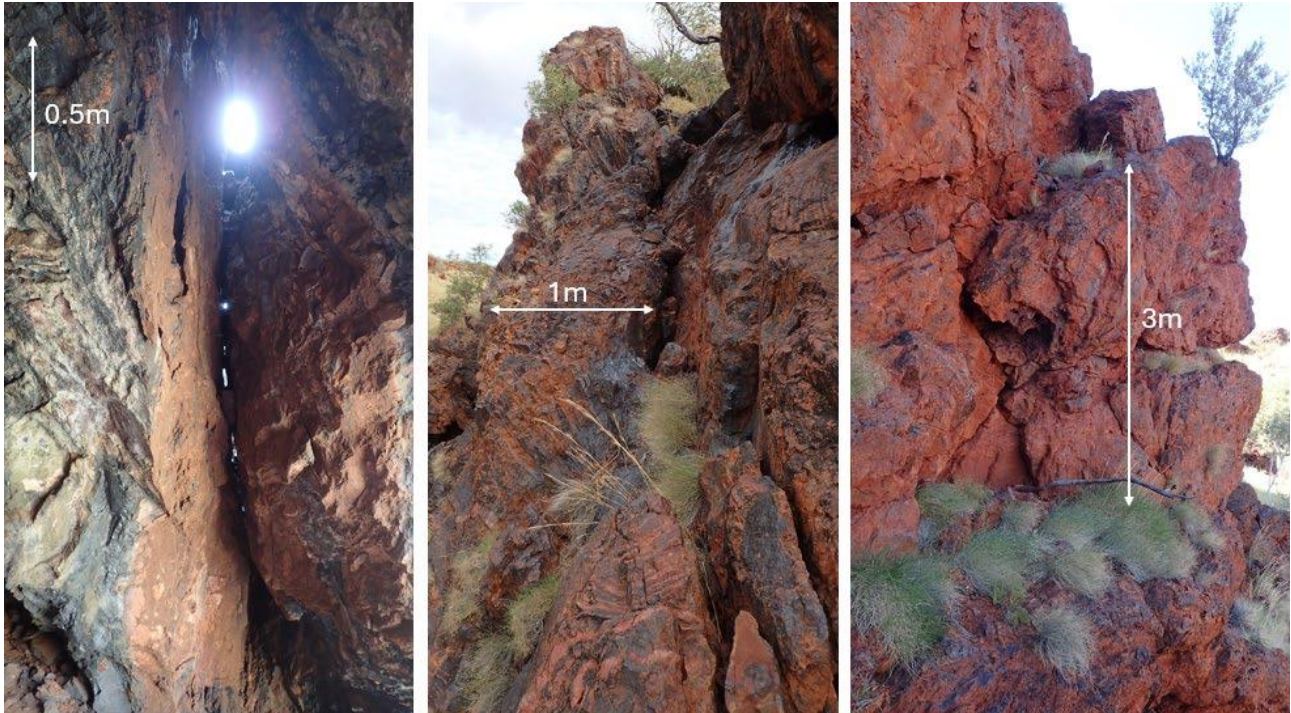
Figure 10 – Examples of separated arches. The left and centre photos are the same separating defect, viewed from the inside (left) and the outside above the cave entrance (centre). In the centre photo the cave entrance is below and to the left. The right photo is another separating defect, viewed from the side of the cave with the entrance around the outcrop to the right.
