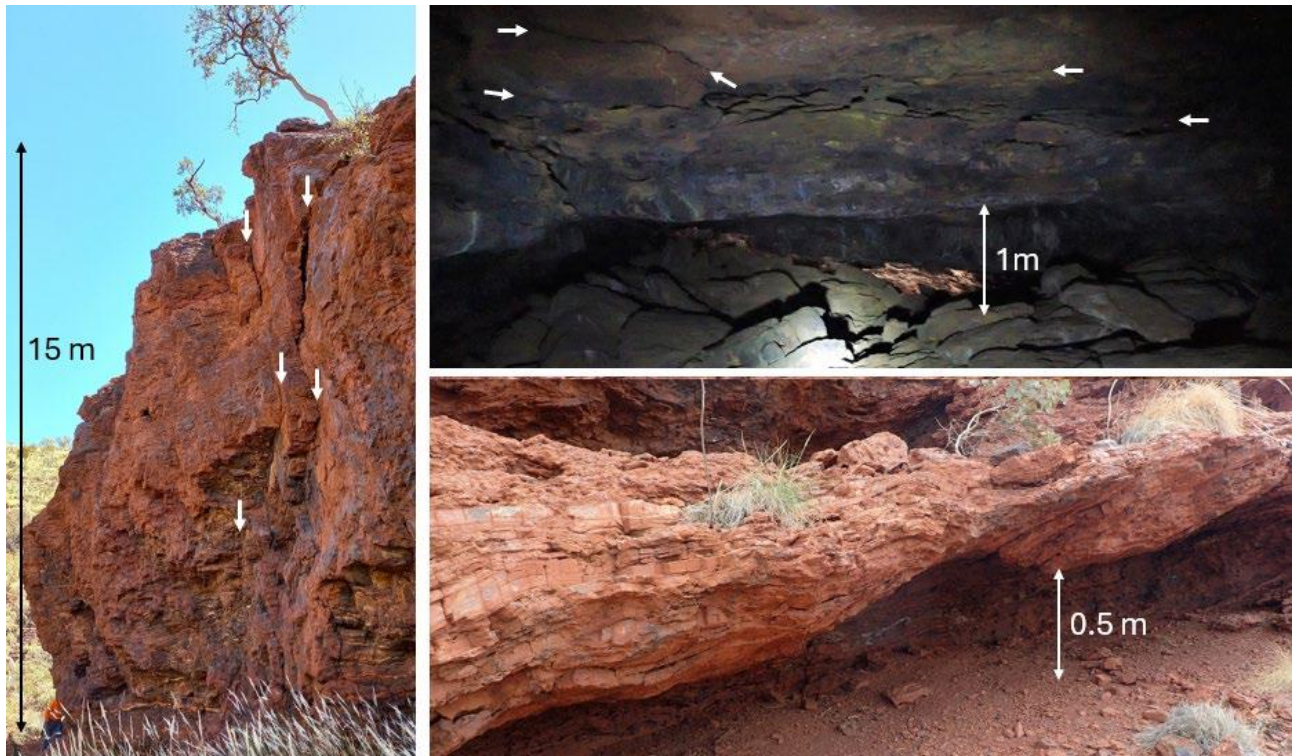
Figure 12 - Examples of potential collapse hazards including escarpment-parallel joints (left), and roof-parallel open joints (top right) and bedding partings (bottom right)
