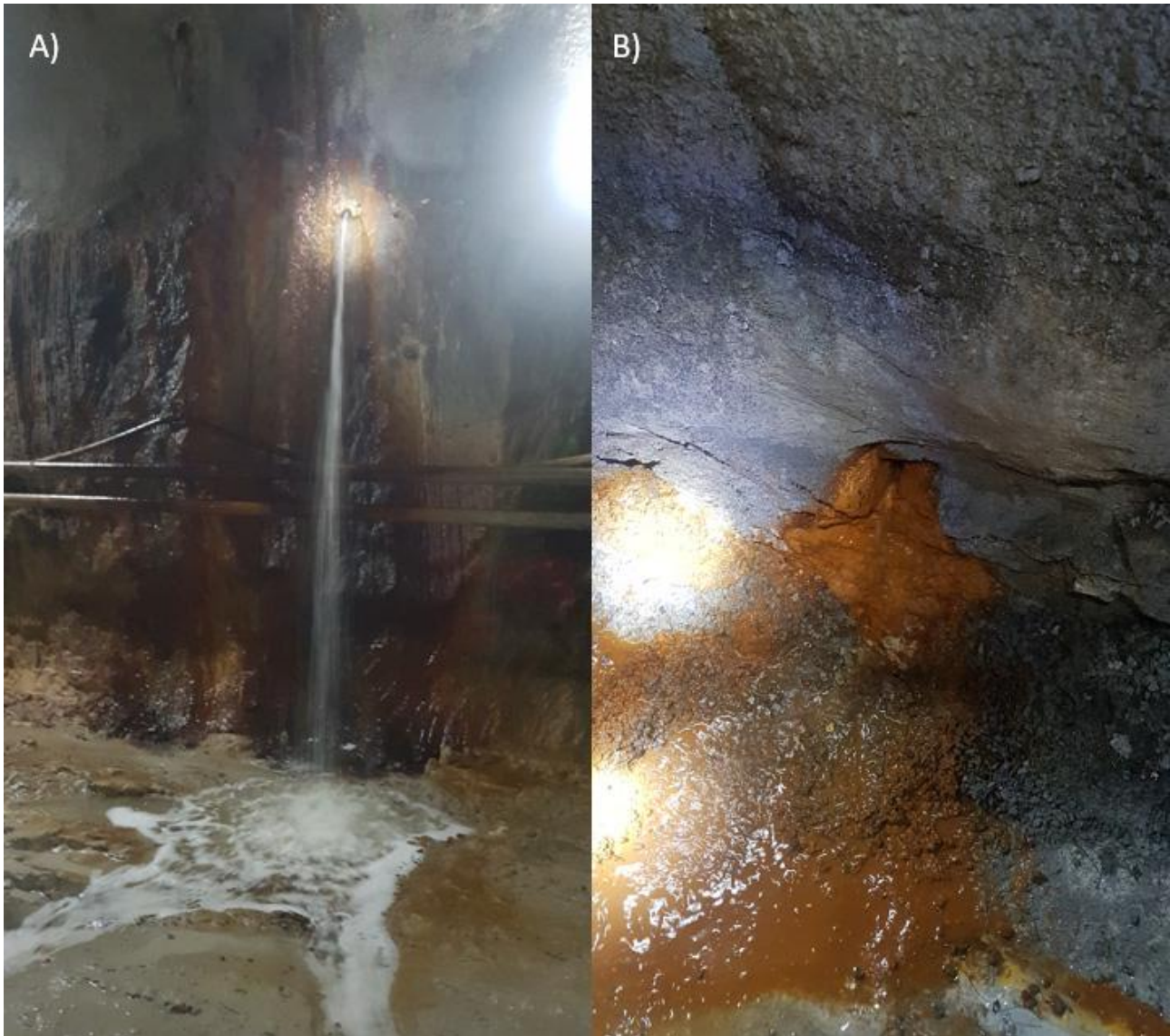
Figure 4: a) flow of water from structure in M8 tunnel with iron precipitation beginning to develop. b) bacterial sludge beginning to develop in association with flowing water in M8 tunnel.
