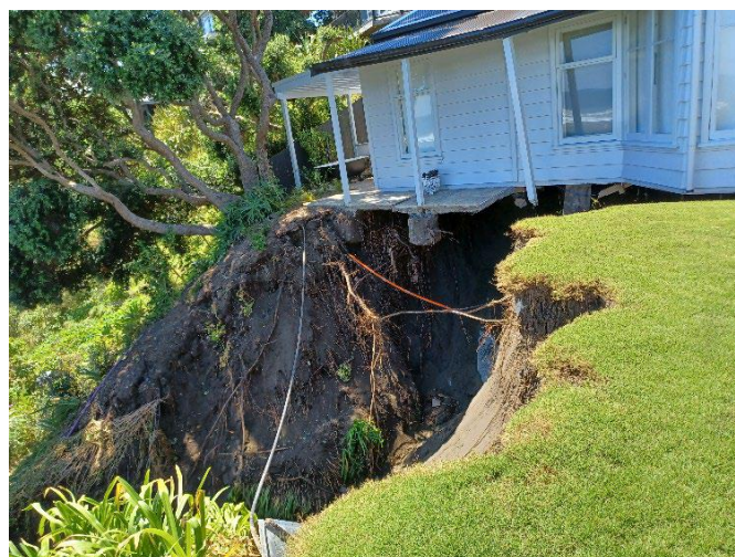
Figure 8: Photograph of a landslide undermining a timber framed dwelling. Leading edge of the dwelling is undermined by approximately 3 m.
