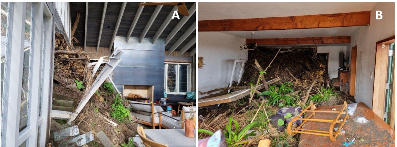
Figure 5: (A) Landslide debris entering into the living room of dwelling by penetrating windows and wall. Dwelling is encased in debris as evidenced by debris visible through window in background. (B) Photograph of the inside of a dwelling which landslide debris has entered. In the background of the image, covered in debris, is the kitchen, the foreground contains the living room.
