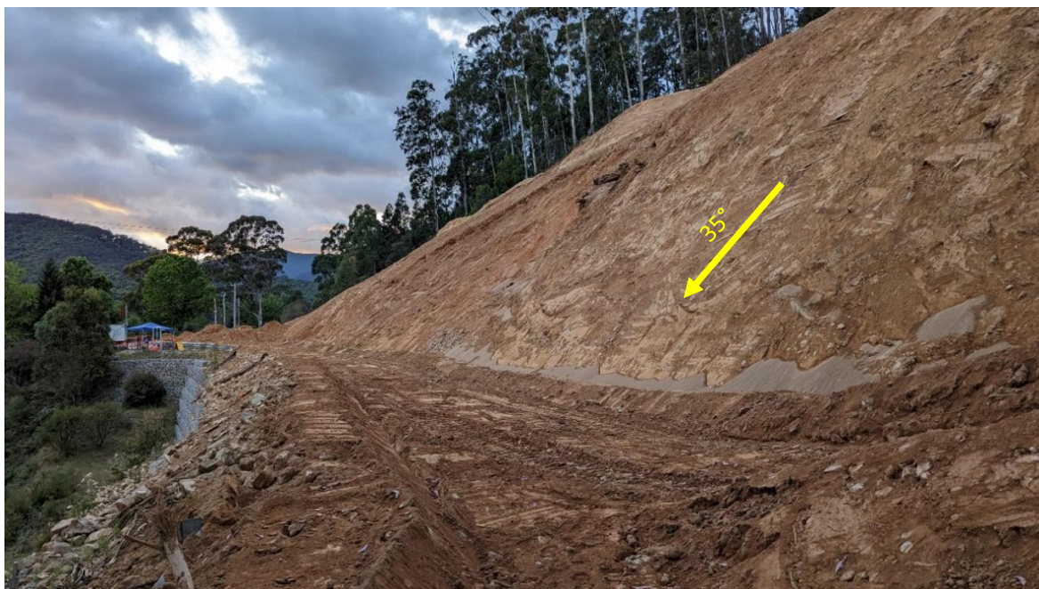
Figure 6: Loose debris at toe of slope, 13 February 2023
