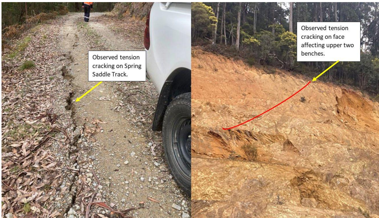
Figure 3: Left: Cracking observed on Spring Saddle Track, 28 September 2022. Right: Cracking observed in face of batter, 5 October 2022
