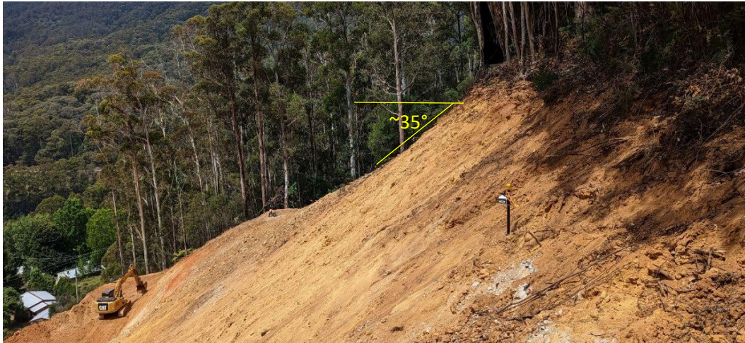
Figure 5: Crest of landslide, 12 January 2023 taken from Spring Saddle Track. Excavation has cut back to in situ material.
