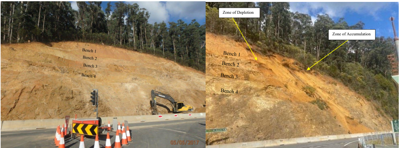
Figure 2: Left: Road Batter in May 2017 at completion of excavation. Right: Road Batter on 8 October 2022 following landslide initiation
