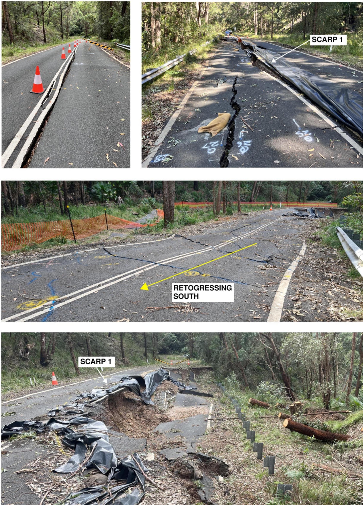
Figure 4: Photos showing the development of the Garie Road landslide. Top left - vertical and horizontal displacement along road centreline (30 March 2022). Top right - significant progression of the deformation (4 April 2022). Middle - landslide retrogressed south (early July 2022). Bottom - Scarp 1 condition (July 2022).
