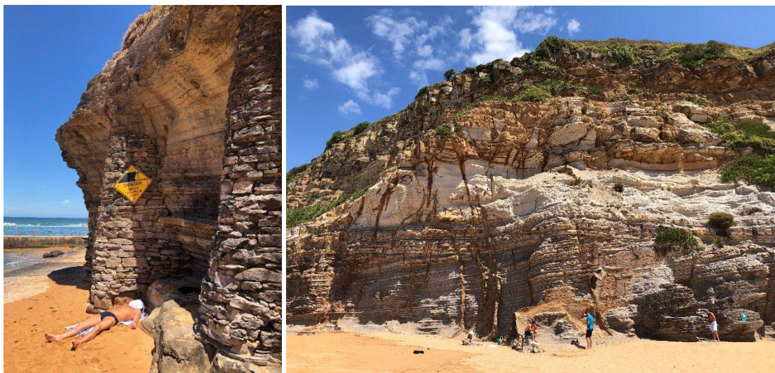
Figure 8: Examples of apparent disregard or unawareness of rockfall hazards, despite signage.
