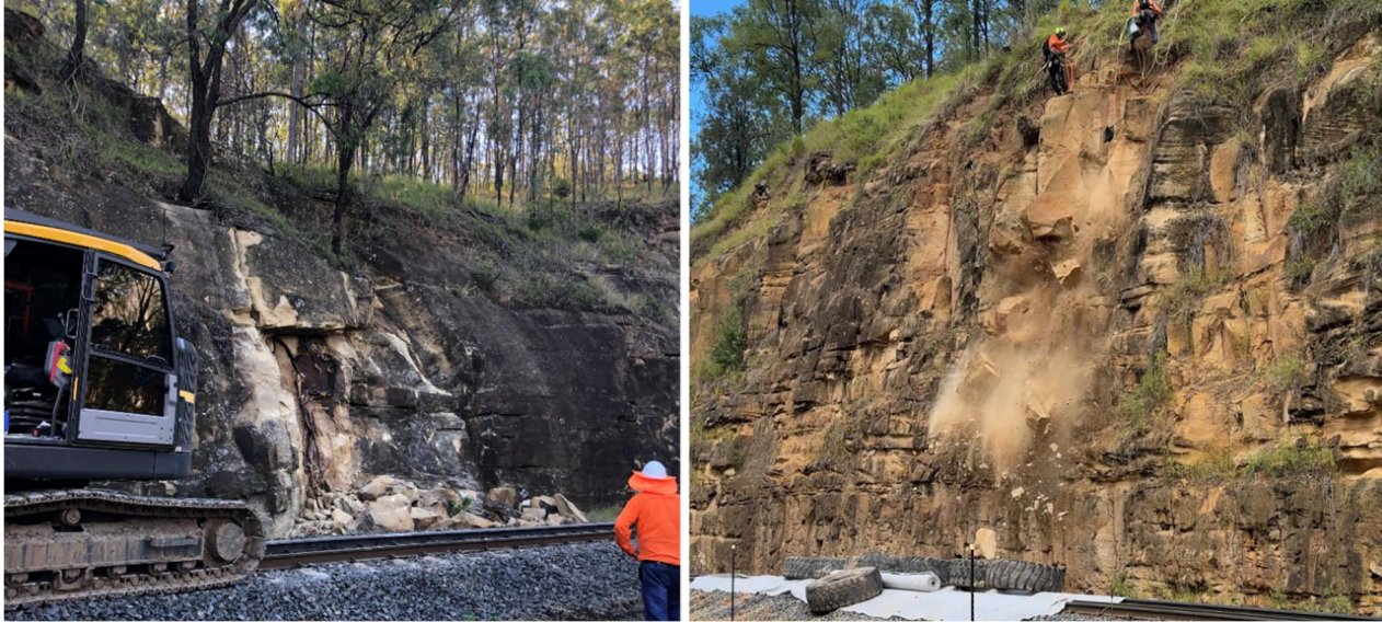
Figure 9: (Left) Rockfalls induced by root jacking, trimming and poisoning of critical vegetation is often utilised. (Right) Roped access assessment and the use of air bags to remove large localised blocks from the slope face.
