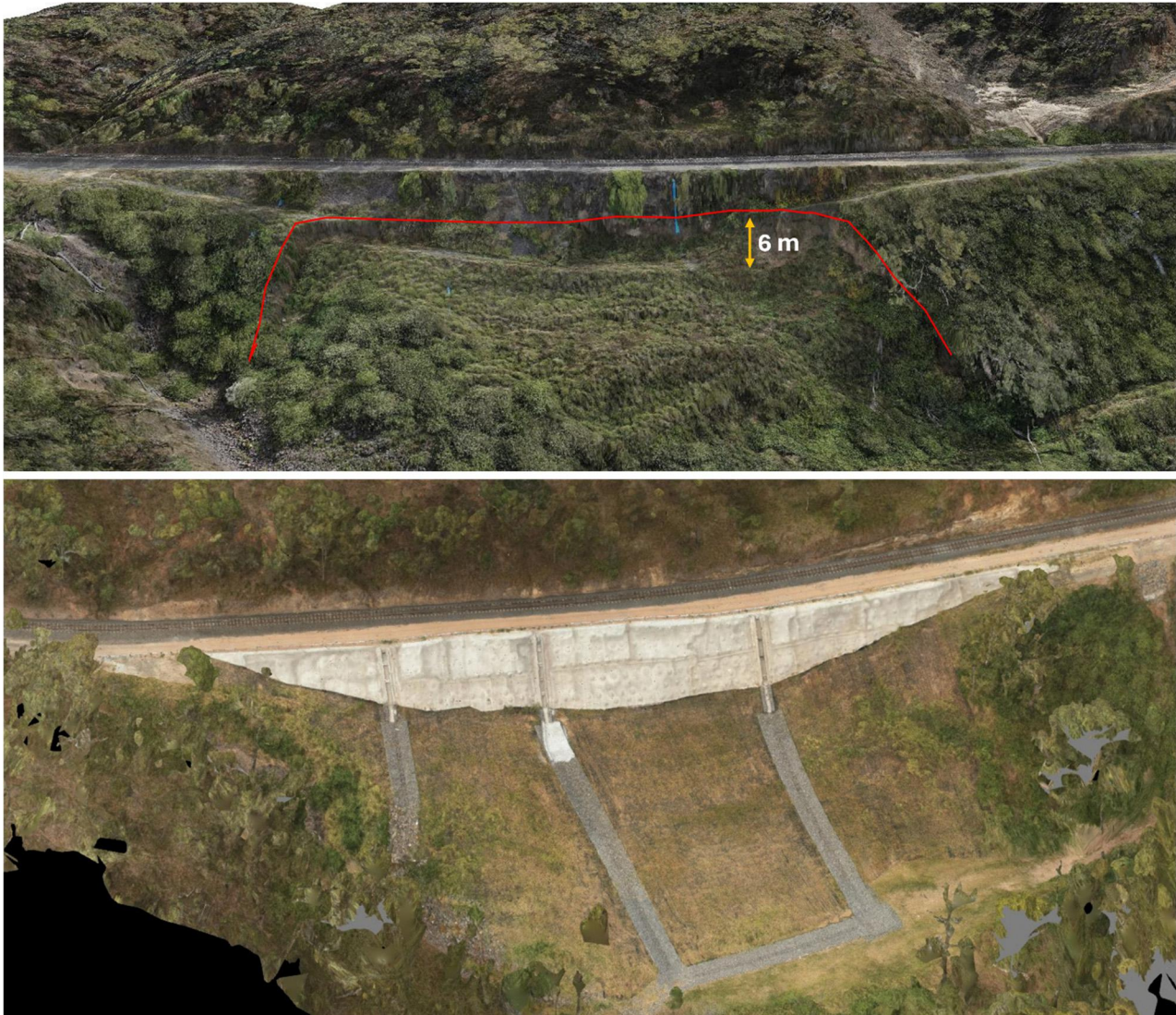
Figure 11: (Top) Reactivation of an existing failure at CH. 141.1 km resulted in the mid-slope access road experiencing 6 m downwards displacement. (Bottom) Post construction condition of the slope following remedial works undertaken in 2023.
