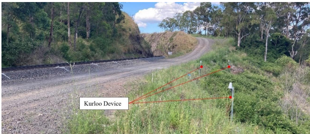
Figure 6: Kurloo instrumentation embankment monitoring
