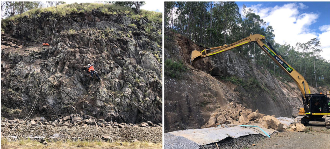
Figure 10: (Left) Extensive scaling via roped access and the use of hand tools. (Right) Mechanical scaling of larger zones of problematic rock mass via long reach excavator.
