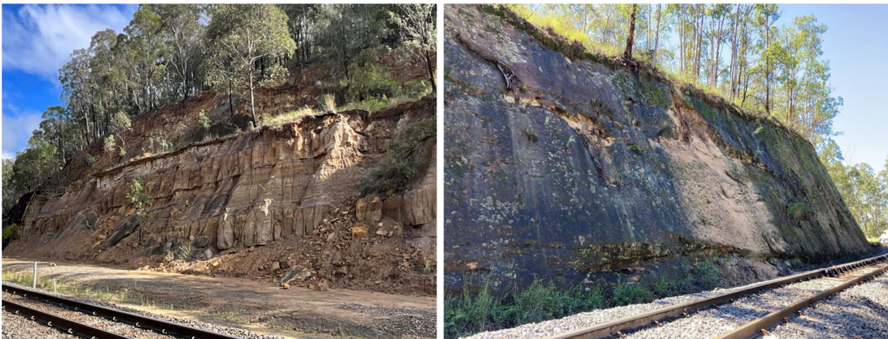
Figure 5: Typical rail cuttings in the Koukandowie Formation (left) and Gatton Sandstone (right)
