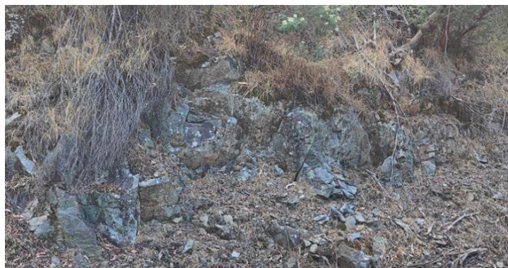
Figure 7: View of a jointed BEDROCK1 on Bogong High Plains Road Ch. 13.88 km.
