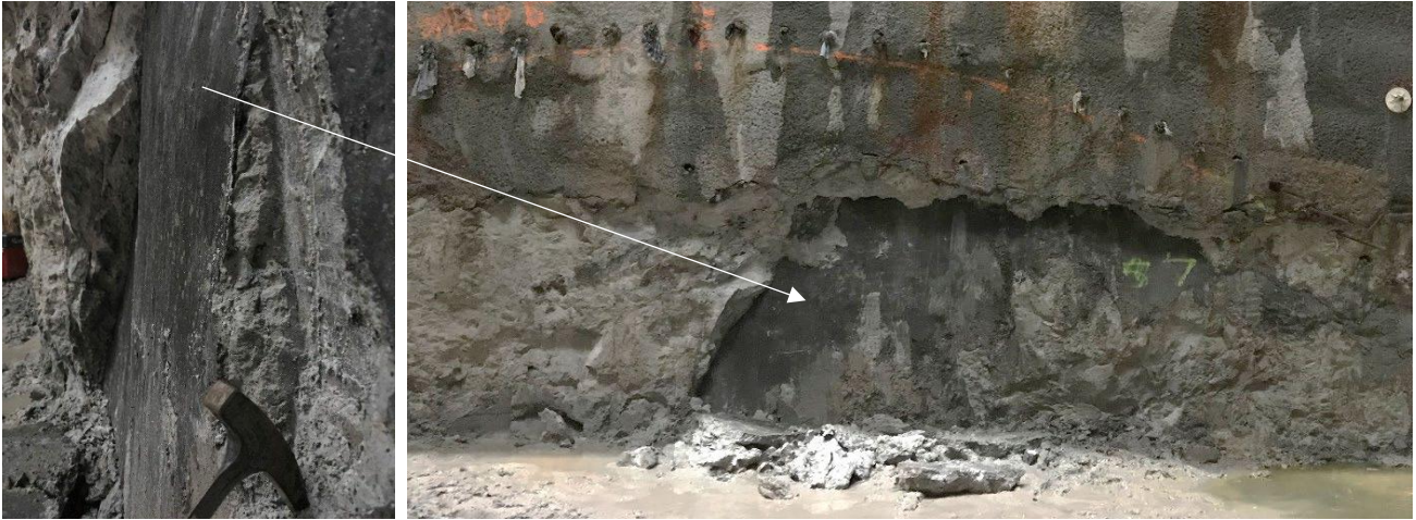
Figure 4: Subvertical shear daylighting in shaft wall at the crown level of the crosscut portal. Highly altered sandy clay breccia and gouge breaking away from the planar, slickensided subvertical shear at rear. Material was readily disaggregated by hand.
