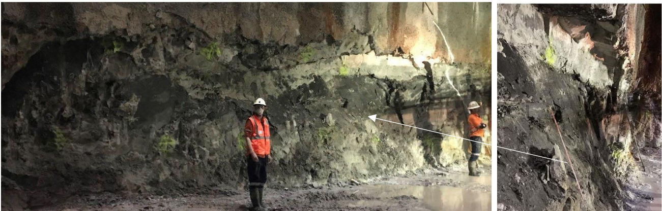
Figure 5: Subsequent excavation lift (approx. -20 mRL) where steeply dipping shears daylighted approximately 2.5 m vertically beneath initial plane. Note undulating defect surface and undercutting of wall along discrete sub horizontal joints
