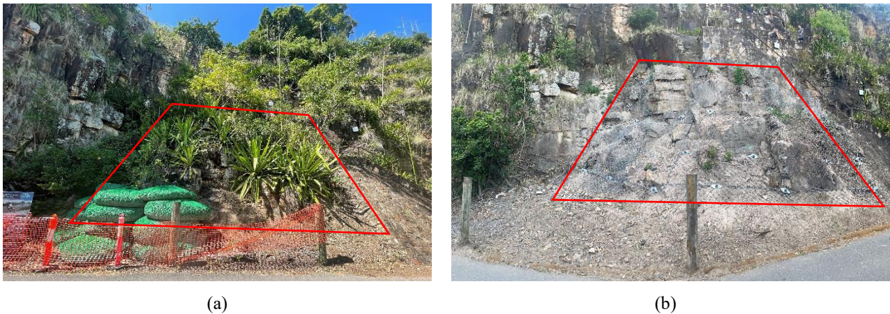
Figure 6: High-capacity wire rope mesh remediation (a) prior to remediation, (b) post remediation
