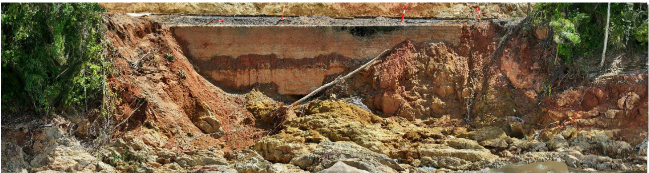
Figure 4: Ground-based field photo of the affected section of the downslope embankment.
