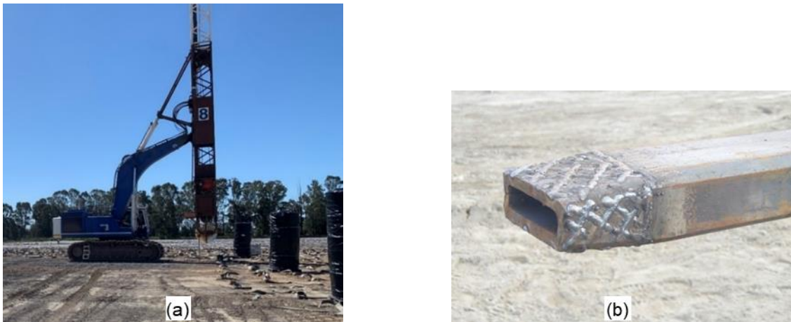
Figure 3: (a) Typical rig setup and (b) Example of mandrel used to install the wick drains
