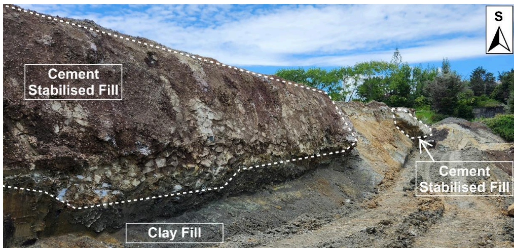
Figure 4: Blocks of cement stabilised fill encountered at NAL 147.145 km.
