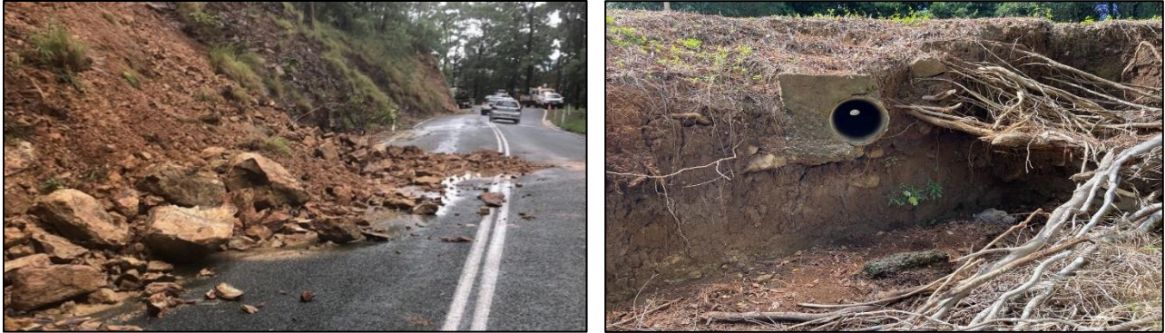
Figure 3: Example failure types Images from the REPA and Betterment Package, upslope site on left and downslope site on right.
