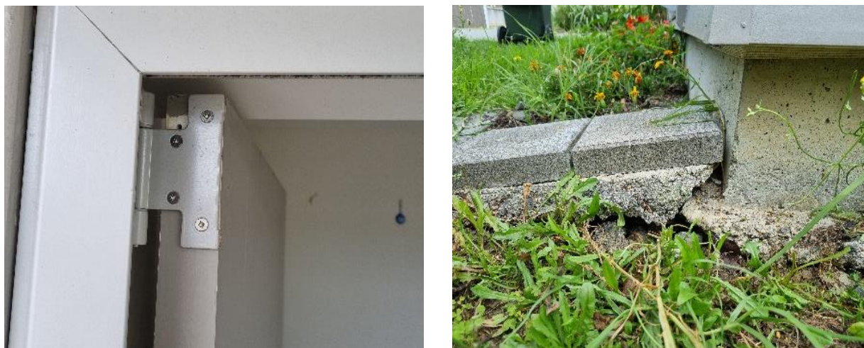
Figure 2: (a) Adjusted door hinge showing clear signs of movement and (b) Garden edging detached from slab and settlement adjacent to pile locations
