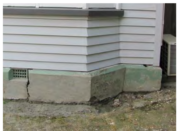
Figure 6: Open cracks on either side of a rotating section of concrete ring beam foundations
