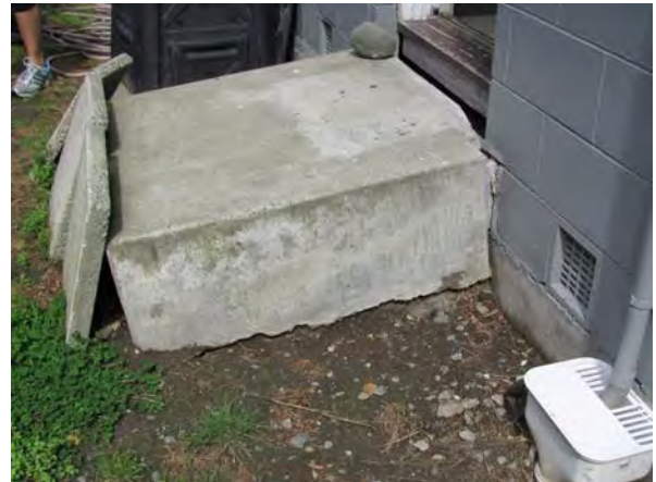
Figure 5: Differential settlement of a doorstep
