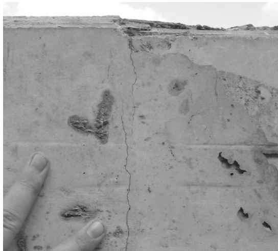
Figure 2: Typical concrete shrinkage crack
