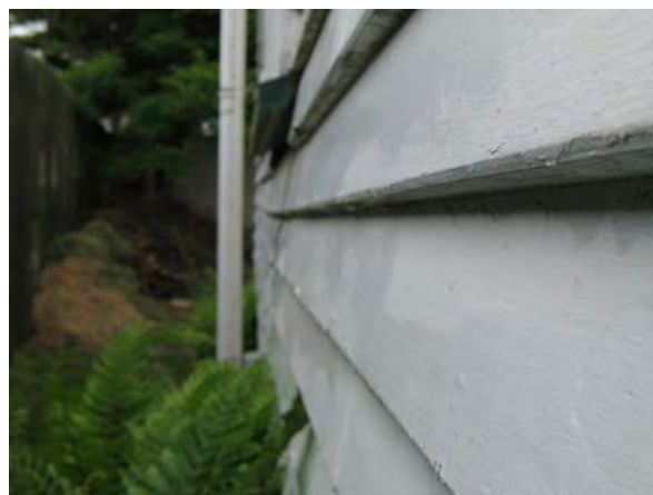
Figure 9: dip in weatherboards directly above the location of a join in the foundation
