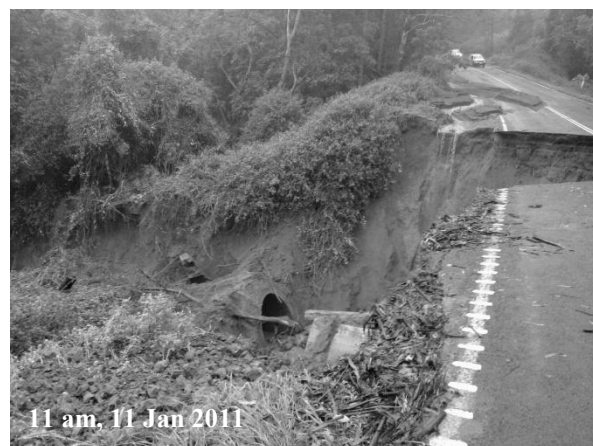
Figure 9. Heavy downstream scour
