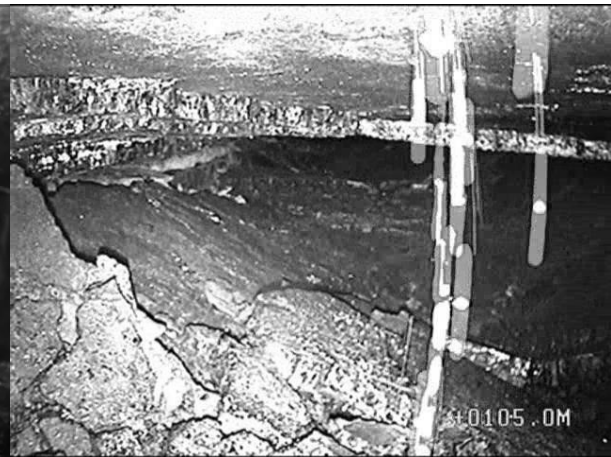
Figure 3b: Roof Collapse
