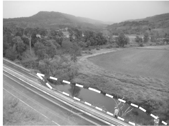
Figure 2. View of failure from crest of roadcut
