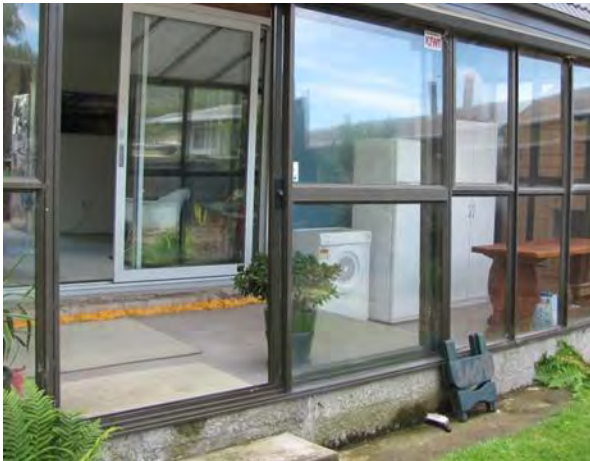
Figure 4: Vertical step where there wasn't meant to be one, between the conservatory and the house.
