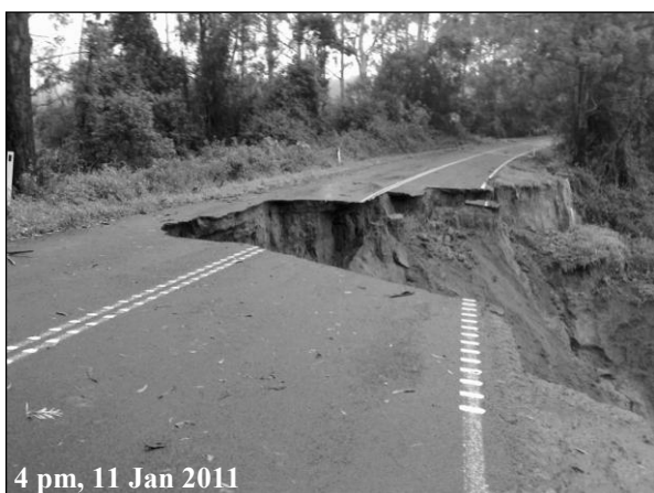
Figure 9. Failure extended into the adjacent lane
