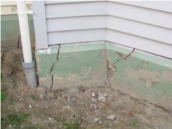
Figure 1: Typical cracking of concrete ring beam foundations
