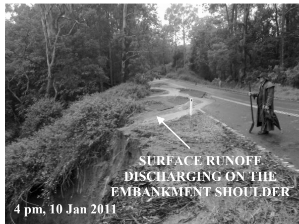
Figure 7. Loss of embankment slope
