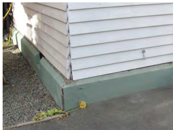
Figure 8: 20mm displacement between the concrete ring beam and the timber framing and cladding
