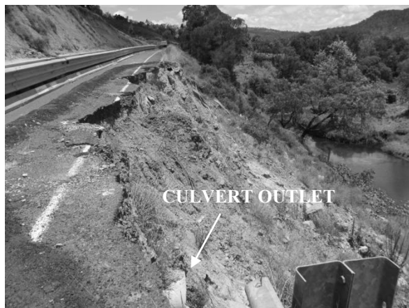
Figure 3. Failure extended into the traffic lane. Note the culvert outlet discharging water onto the slope
