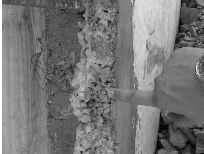
Figure 1: Concrete 'honeycomb' structure within diversion structure wall
