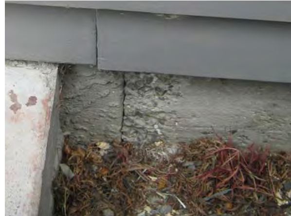
Figure 2: Typical spalling at a join between two foundations
