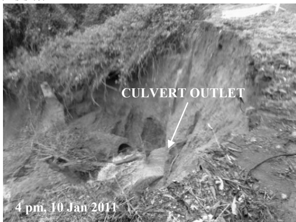
Figure 6. Failure of embankment slope around culvert
