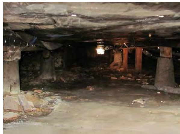
Figure 3: Sunken piles and wavy bearers
