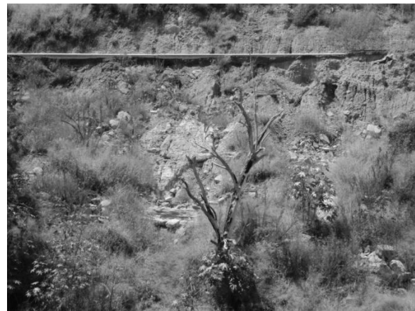
Figure 4. View of failure from toe of slope adjacent to creek
