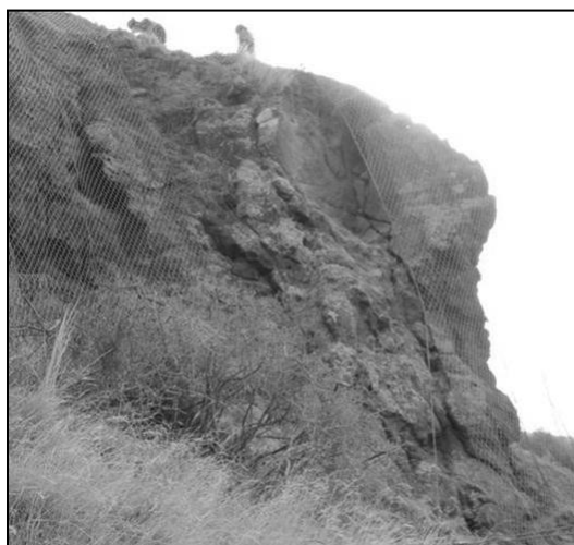
Photograph 1. Meshing of failed / failing bluff (High Risk)
