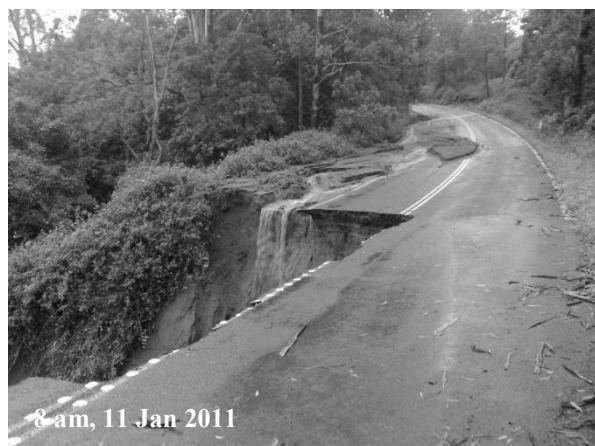
Figure 8. Damage extended to the centre line
