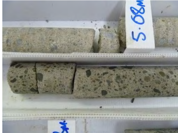
Figure 3. Typical core cracks
