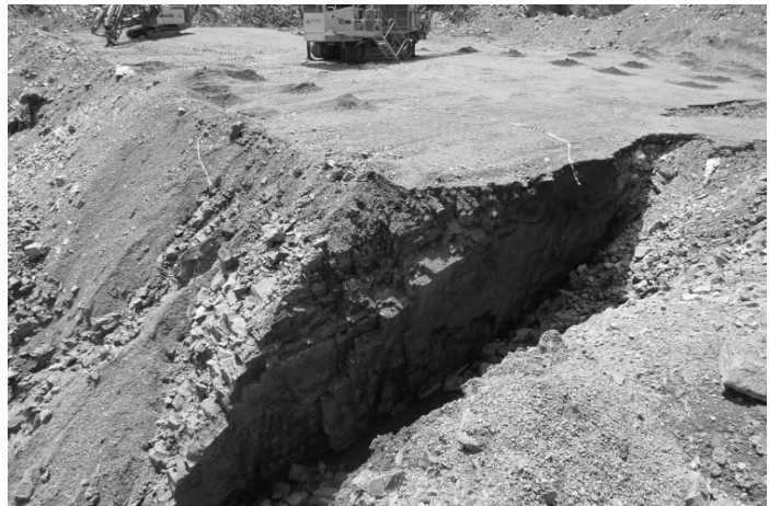
Figures 5, Stope fill subsidence and washout after heavy rainfall
