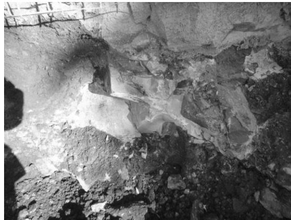
Figure 2: Grout Losses within Basalt and Colluvium in Cut 18
