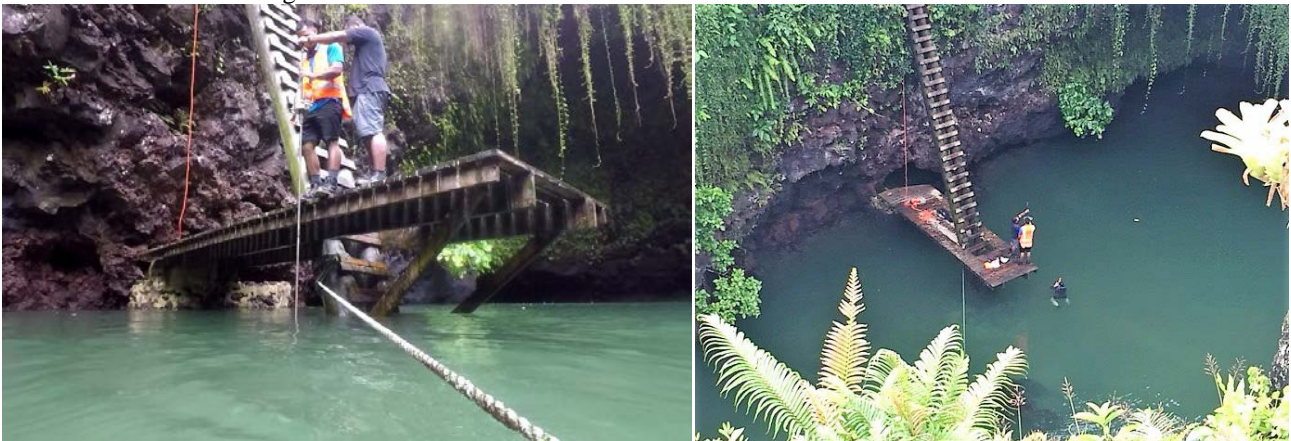
Figure 3: Undertaking Scala penetrometer testing from the platform at the base of the ladder and evaluating the base of the trench through swimming.
