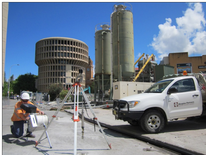
Figure 2: Grout plant set up in Newcastle CBD, with downhole camera being deployed in to a bore to assess the grouting operations
