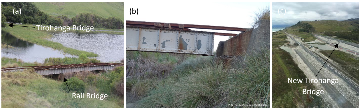
Figure 7: a) Flooding of the bridge site after earthquake, b) Rail Bridge unseated girder, c) new Tirohanga road and Rail bridges (photos courtesy of NCTIR and GEER)
