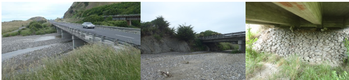
Figure 2: Kekerengu River Bridge, bridge overview looking south (left); north abutment on rock (middle); south abutment on soil (right) prior to earthquake
