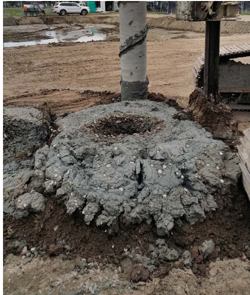
Figure 3 Typical Heave from Stone Column Installation
