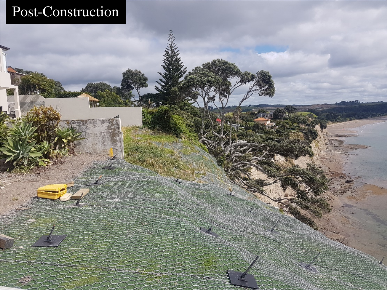
Figure 4: Pre-and post-construction photos of the Site A. Remediation was undertaken in two stages across the property boundary a few months apart, notice the rapid revegetation of the distal slope
