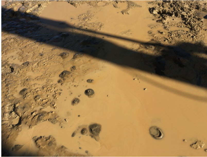
Figure 4: Sand boil formation at base of foundation excavation (August 2017).
