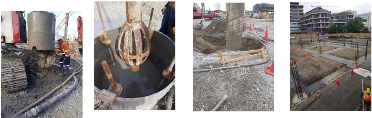
Photographs from Left – Pile Rotary Auger Bucket, Pile Temporary Casing showing drilling mud with Hold down and hold up bars for casing and tremie pipe about to be lowered into hole, Casing Withdrawal, Completed piles with site concrete for ground beam pour.
