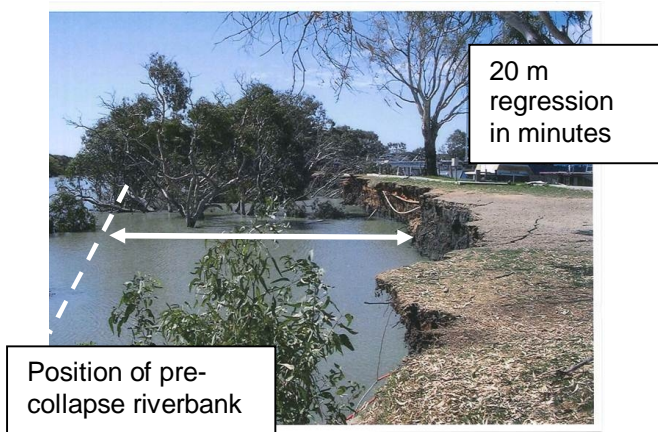
Photograph 1. Riverbank Collapse at Long Island Marina, Murray Bridge.
