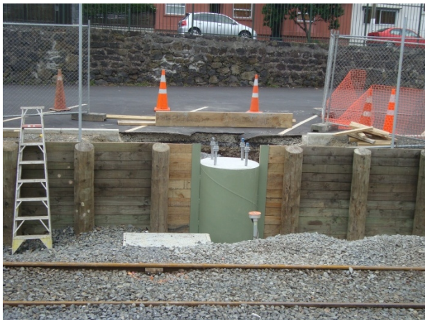
Figure 3. A twin-track cantilever mast foundation at Mt Eden.
