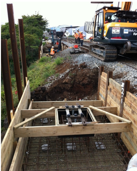
Figure 2. A pad foundation being constructed in a basalt gravel embankment near Morningside.
