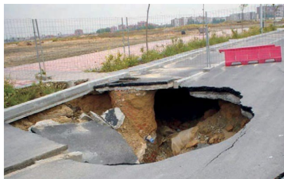
Figure 2. Sinkhole discovered on V-5 roadway, May 2006.
