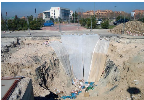
Figure 1. A sinkhole discovered on La Gavia Avenue, situation in March 2018.
