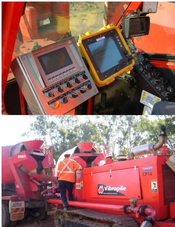
Figure 5. Installation monitoring control and display panels (Top) and concrete truck unloading into concrete pump (Bottom).
