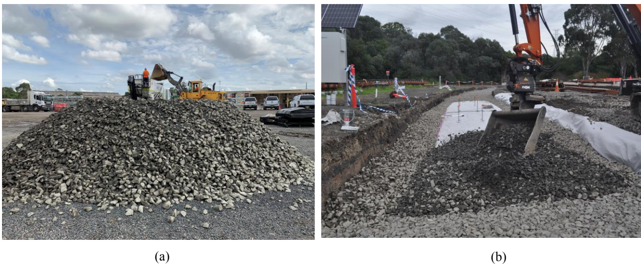
Figure 5: (a) Onsite blended RIBS (b) Placement of RIBS on track at reduced height ( 1 < \text{m} )
