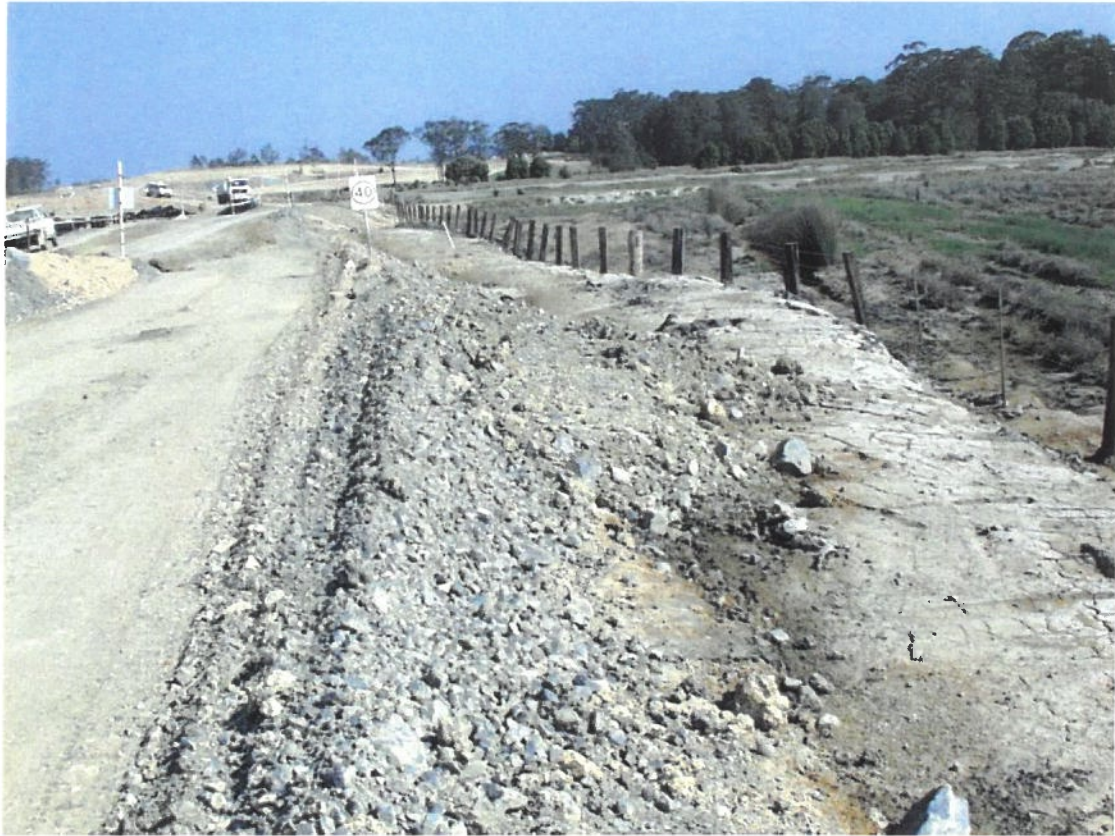
Photo 1: Lateral soil movement adjacent to toe of embankment
