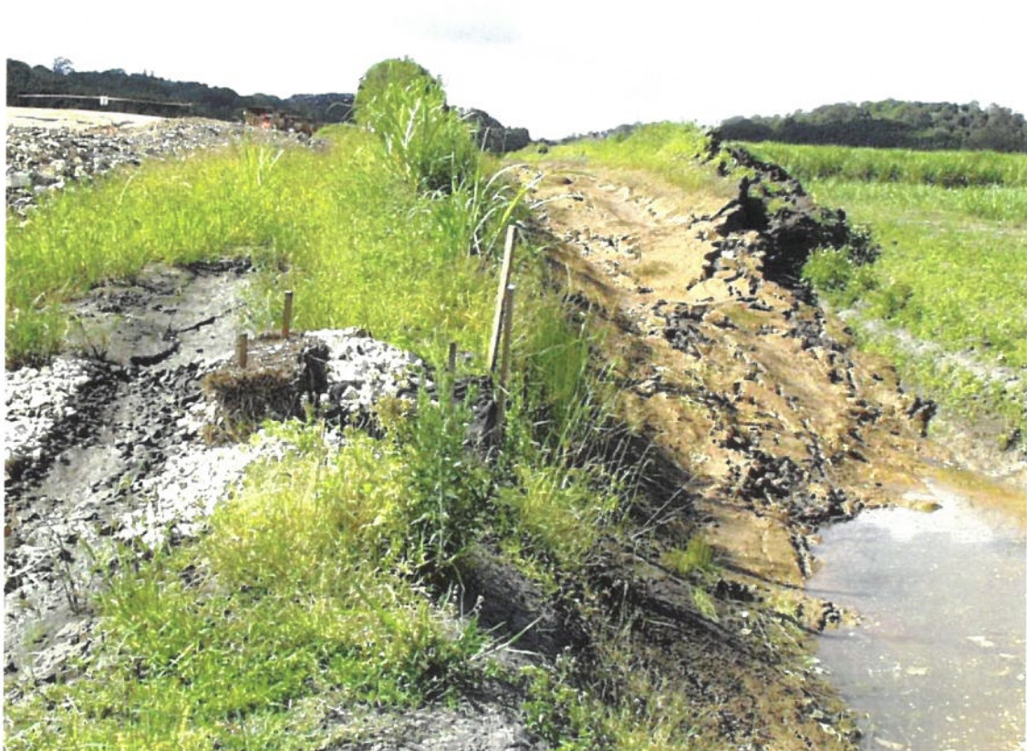
Figure 2: Ground heaving adjacent to toe of embankment
