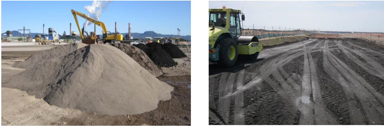
Figure 2: Compaction trial (a) Coal wash and steel furnace slag and (b) Vibration roller
